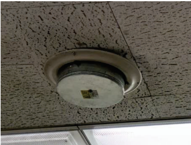
Cap covering non-working HVAC vent in NUSD district office
