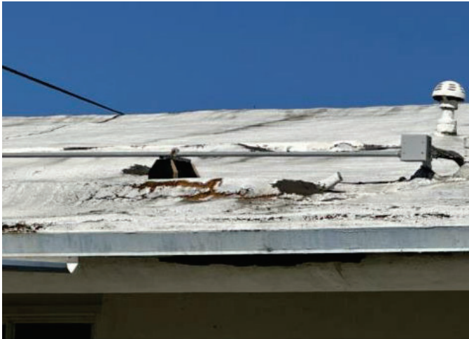
Damage to roof of NUSD district office
