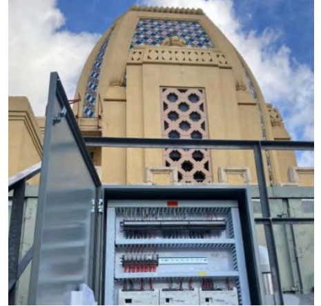
Fox Theater HVAC Controls Replacement
