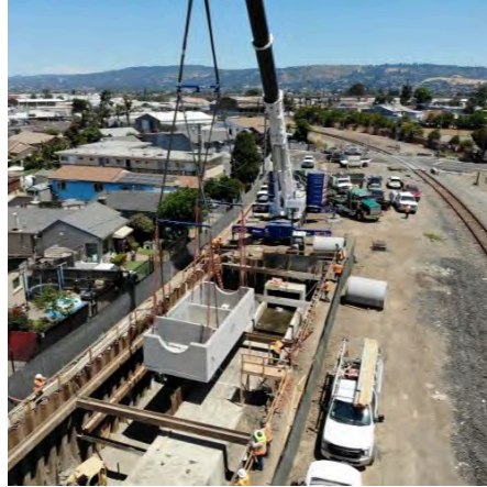
Large Trash Capture Devices At Cary Ave & Mandela Pkwy
