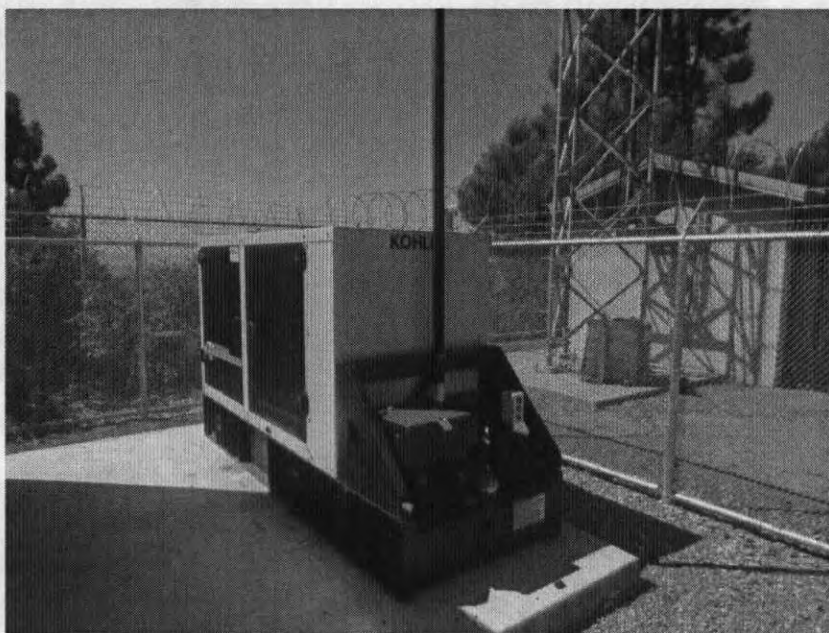
EBRCS Generator at Seneca Reservoir
