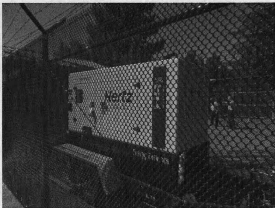
Oakland Fence and portable generator at Seneca site
