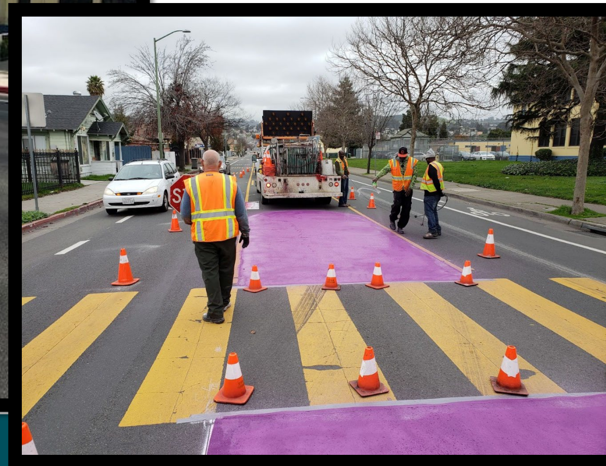
98th and Cherry Safety Improvement Project (near term improvement later installed with concrete)
