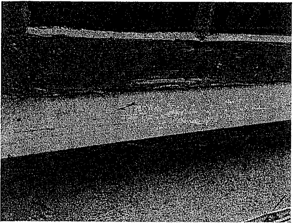
Figures 10, 11 & 12: Pictures of representative samples of damage to windows and doors.
