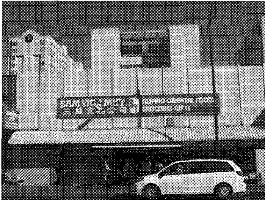
8th Street and Webster: obsolete building design, peeling paint, deteriorated facade.
