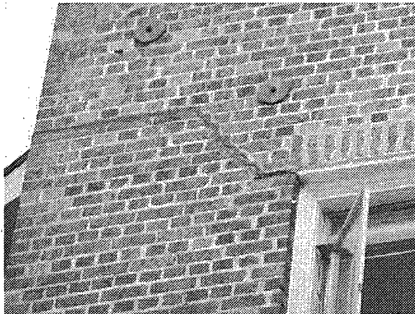
Bay Place and Access Road: cracked masonry wall potentially hazardous in event of earthquake, building vulnerable to serious damage in event of earthquake.
