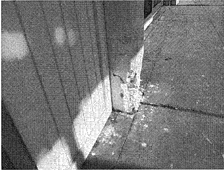
2nd Street and Webster: crumbled and cracked structural support
