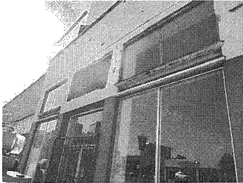
26th and Broadway: peeling paint, dry rot and cracked wall on commercial building apparently due to long-term neglect.
