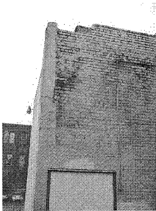
9th Street and Clay: unreinforced masonry building vulnerable to serious damage from seismic events, cracked and deteriorated wall potentially hazardous in event of earthquake, peeling paint.
