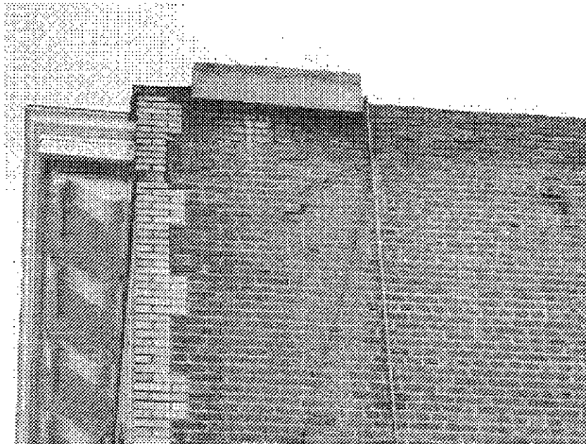
26th Street and Telegraph: partially reinforced masonry building vulnerable to serious damage from seismic events, cracked masonry wall potentially hazardous in event of earthquake.
