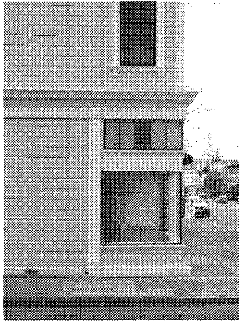
25th Street and Telegraph: structural alignment problem observed at ground floor.
