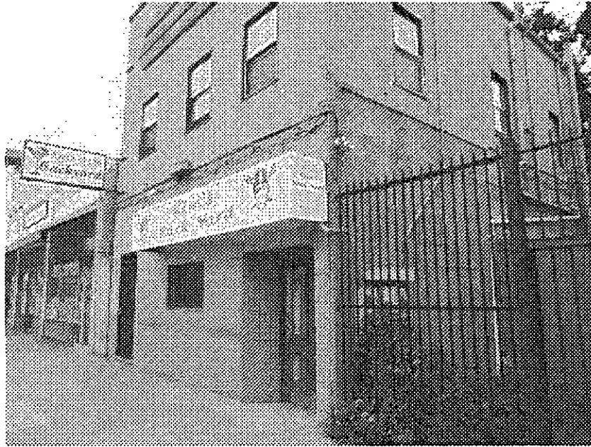
25th Street and Telegraph: dry rot peeling paint and cracked wall apparently due to long-term neglect ,
