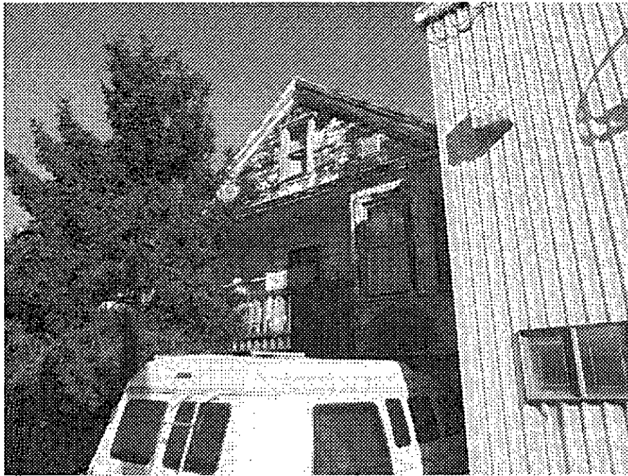
4th Street and Bmsh: serious deterioration and dilapidation apparently due to long-term neglect, deteriorated siding and eaves, peeling paint, dry rot.
