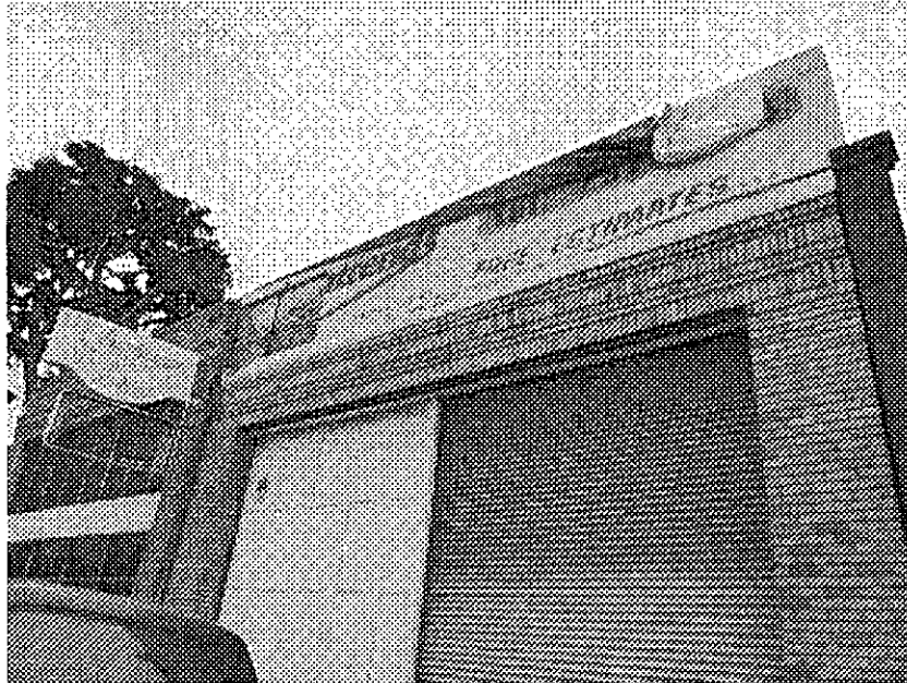
24th Street and Waverly: unreinforced masonry building vulnerable to serious damage from seismic events, building potentially hazardous in event of earthquake, deteriorated facade.
