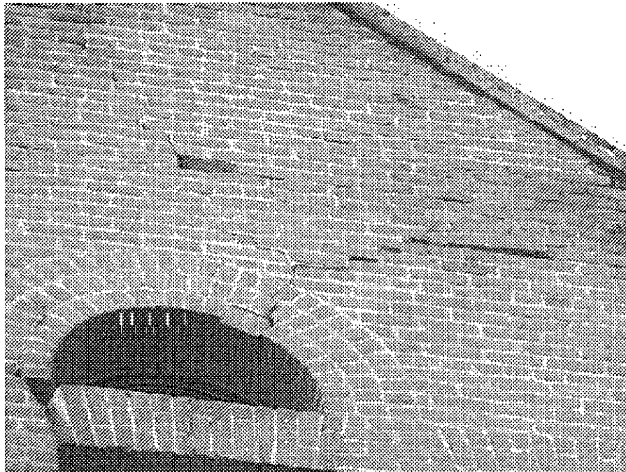
Grand and Valdez (close up of above): cracked and deteriorated masonry wall potentially hazardous in event of earthquake, building vulnerable to serious damage from seismic events.
