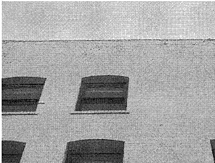
16th Street and Martin Luther King (close up of above): partially reinforced masonry building vulnerable to serious damage from seismic events, cracked and deteriorated masonry wall potentially hazardous in event of earthquake.
