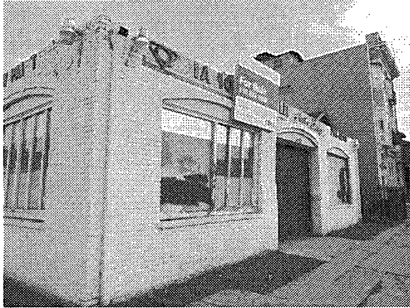
20th Street and Castro: partially reinforced masonry building vulnerable to serious damage from seismic events, potentially hazardous in event of earthquake, vacant and boarded commercial building, graffiti.
