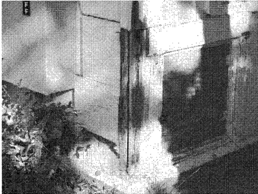
17th Street and Madison: brick foundation causing building to be vulnerable to serious damage in seismic events, deteriorated siding, peeling paint, dry rot.
