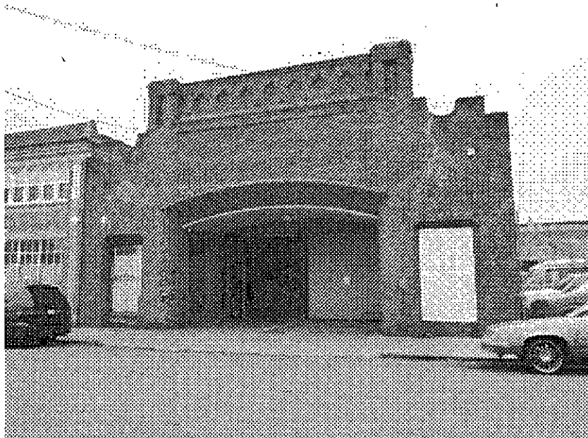
24th Street and Valley: partially reinforced masonry building vulnerable to serious damage from seismic events, cracked wall potentially hazardous in event of earthquake, boarded windows.
