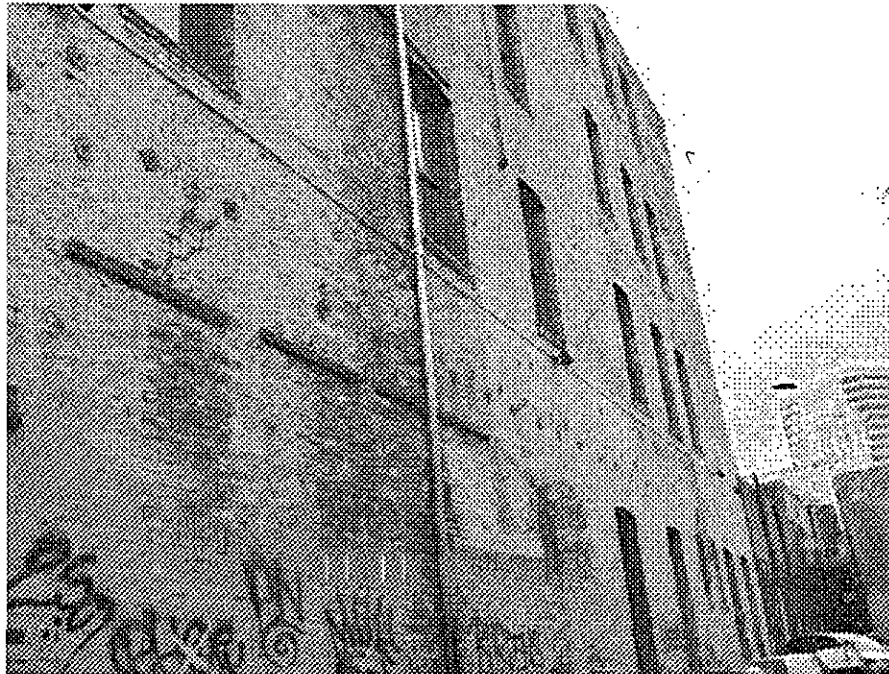
12th Street and Harrison: partially reinforced masonry building vulnerable to serious damage from seismic events, cracked masonry wall potentially hazardous in event of earthquake, graffiti.
