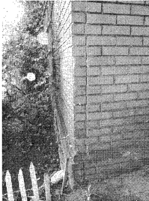
17th Street and Alice (close up of above): cracked masonry at building corner potentially hazardous in event of earthquake, building vulnerable to serious damage in event of earthquake.
