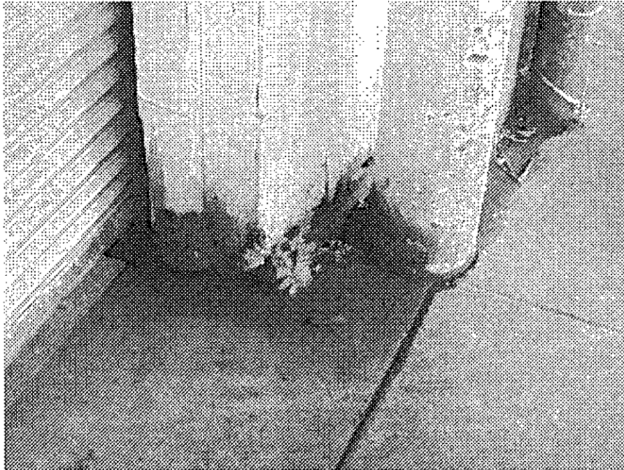
2nd Street and Broadway: deteriorated structural support.
