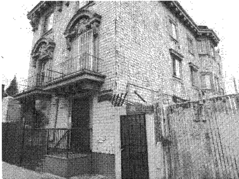
24th Street and Telegraph: serious deterioration and dilapidation apparently due to long-term neglect deteriorated siding, dry rot peeling paint.
