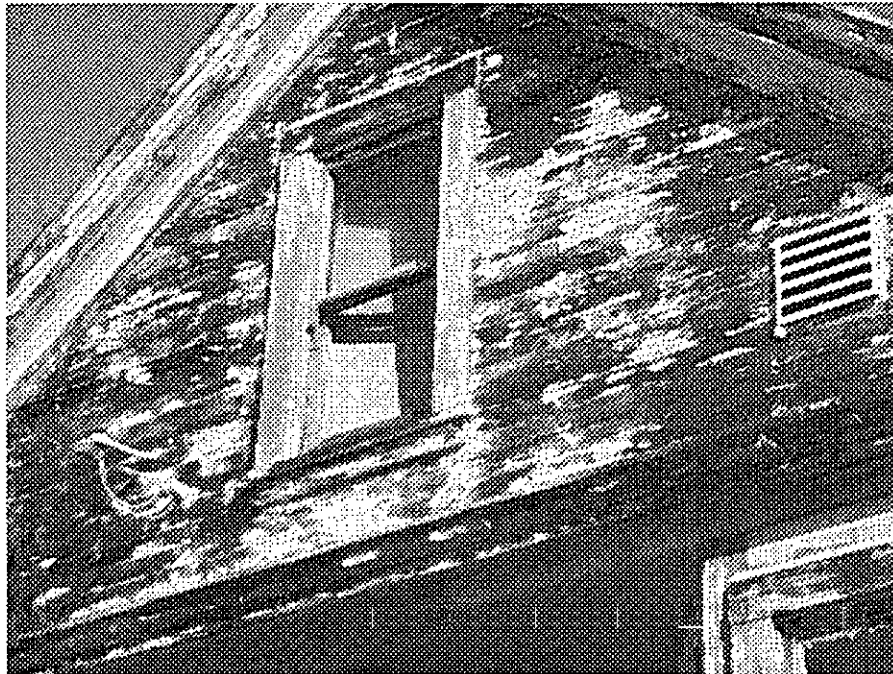
4th Street and Brush (close up of above): missing and boarded window, peeling paint, deteriorated siding and eaves, severe dry rot.
