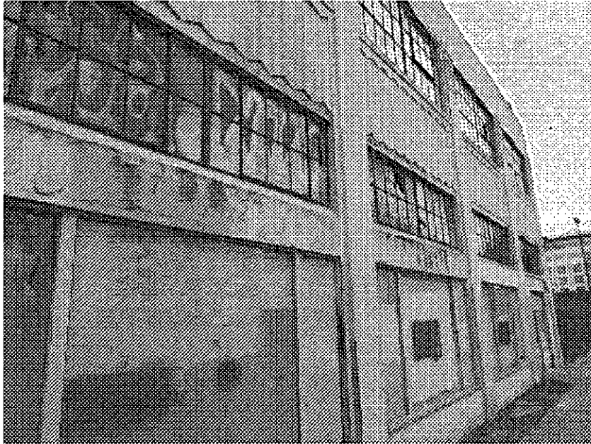
24th Street and Valley: abandoned, vacant commercial building, serious dilapidation apparently due to long-term neglect, broken and boarded windows and doors, cracked walls, graffiti.
