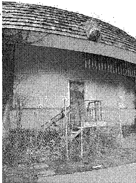
27th Street and Valdez: abandoned, vacant and boarded commercial building, obsolete building design.
