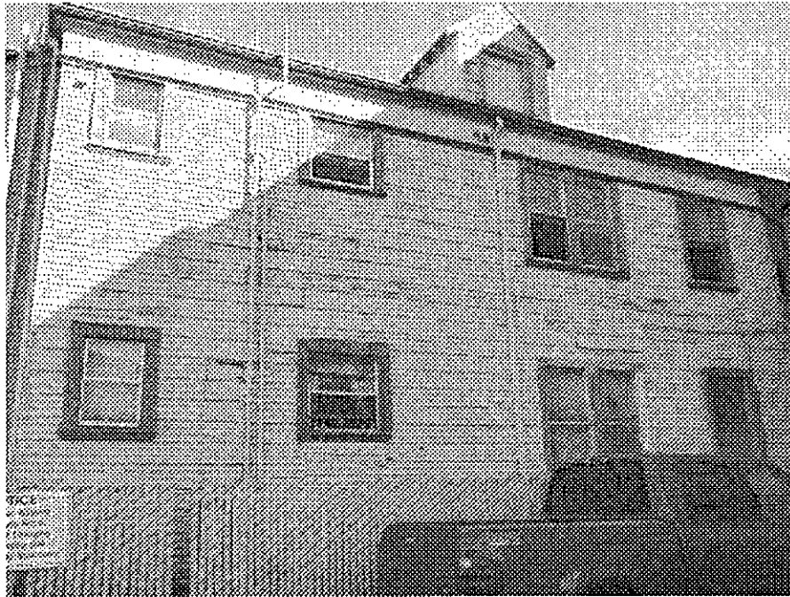
14th Street and Castro: serious deterioration apparently due to long-term neglect missing siding, peeling paint, dry rot.
