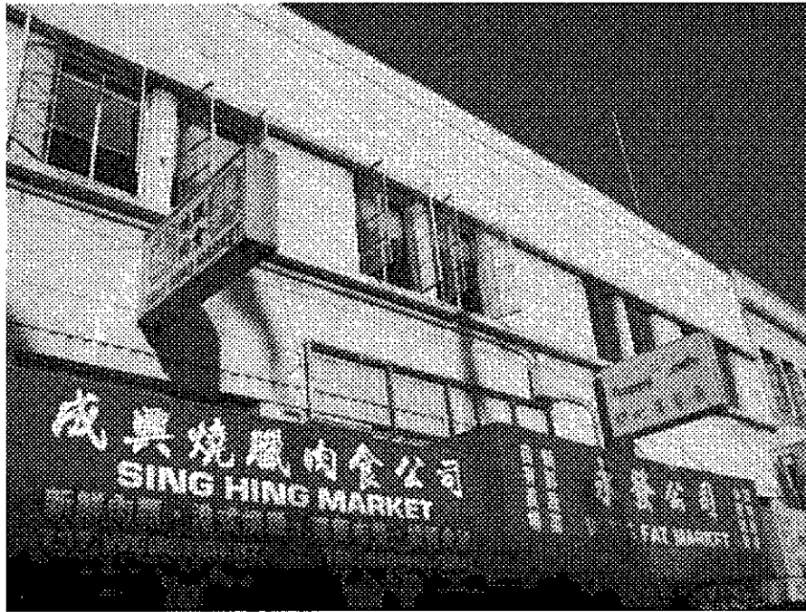
7th Street and Webster: peeling paint, cracked walls.
