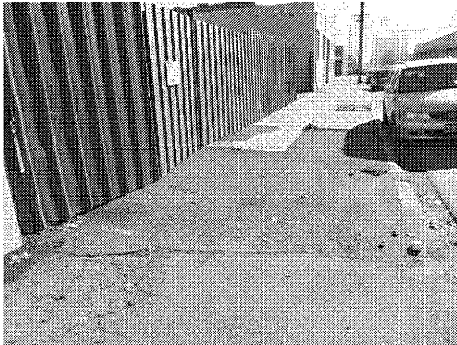
3rd Street and Brush: deteriorated and uneven sidewalk.
