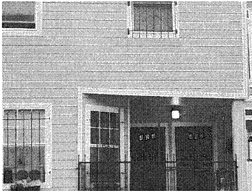
24th Street and Telegraph: sagging building overhang suggests structural alignment problems.
