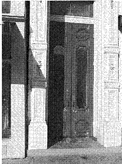
8th Street and Washington: cracked wall and structural alignment problems observed on left side of building, peeling paint.
