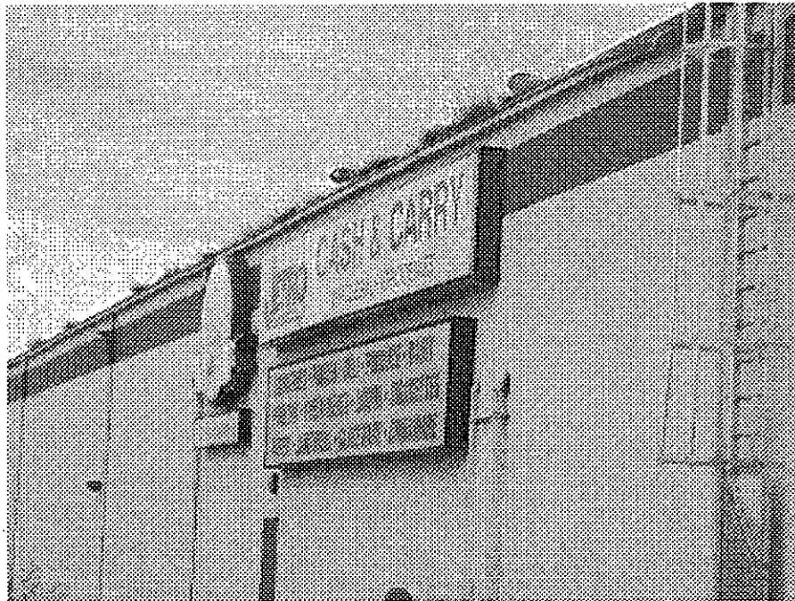
1st Street near Estuary Park: deteriorated roof and gutters likely allowing moisture intrusion, mold contamination and structural wood rot.
