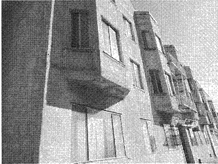
9th Street and Madison: serious deterioration apparently due to long-term neglect peeling paint cracked walls.
