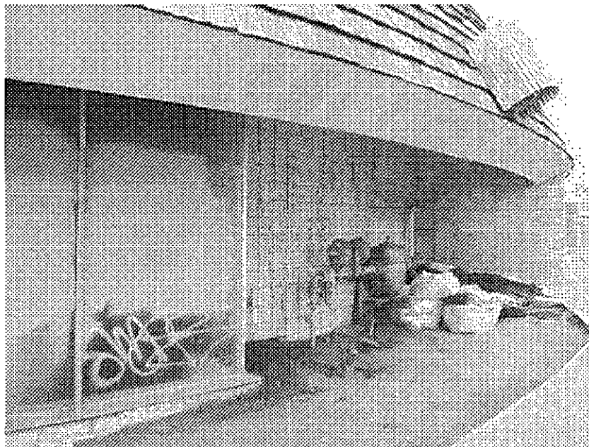
27th Street and Valdez (same building as previous photo): apparent long-term neglect evidenced by vandalism and illegal garbage dumping.
