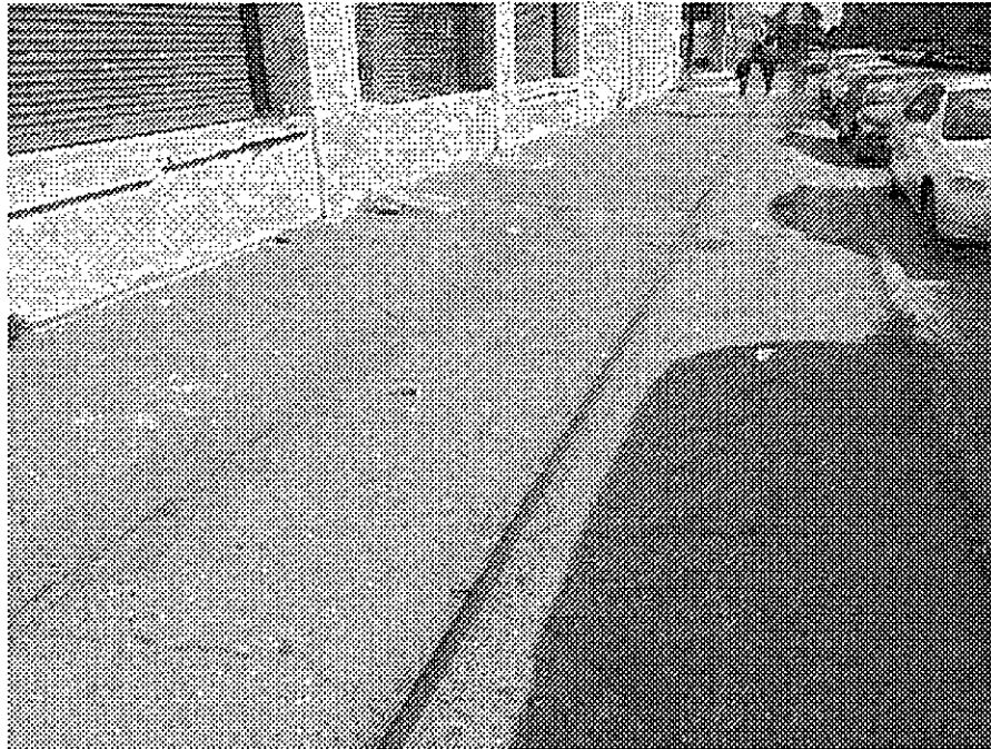
4th Street and Harrison: deteriorated and inadequate sidewalk, abandoned and defunct rail lines.
