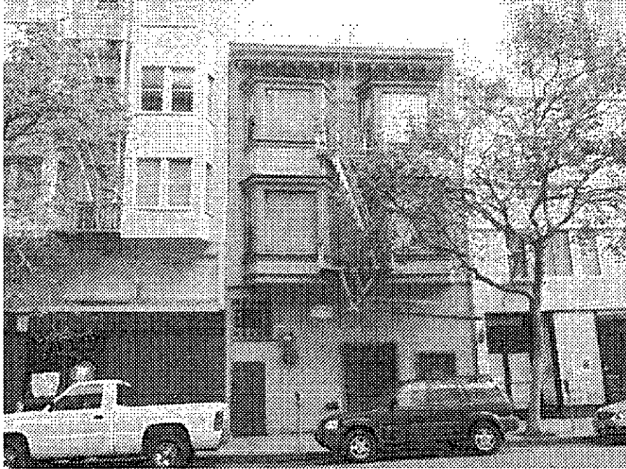
15th Street and Jefferson: peeling paint, deteriorated siding, dry rot,
