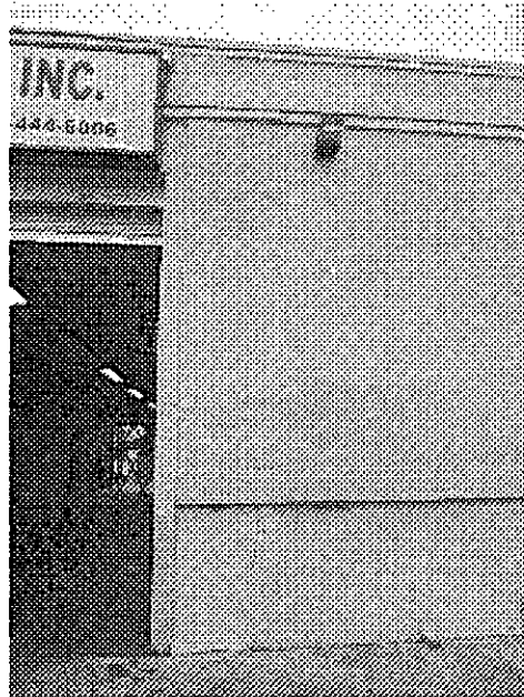
25th Street and Broadway: cracked wall, peeling paint.
