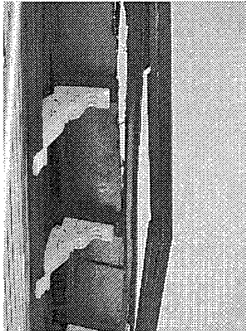
18th Street and Castro: severe eave separation likely allowing moisture intrusion, mold contamination and structural wood rot, eave deterioration.
