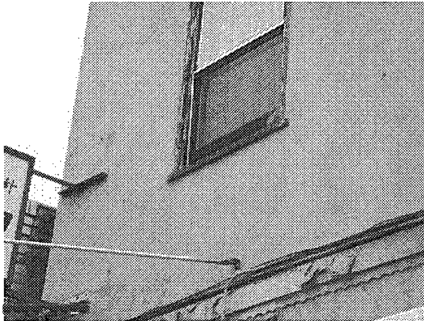
25th Street and Telegraph (close up of above): dry rot, peeling paint cracked wall.
