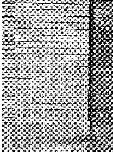
24th Street and Waverly (close up of above): cracked and deteriorated masonry wall potentially hazardous in event of earthquake, building vulnerable to serious damage in event of earthquake.
