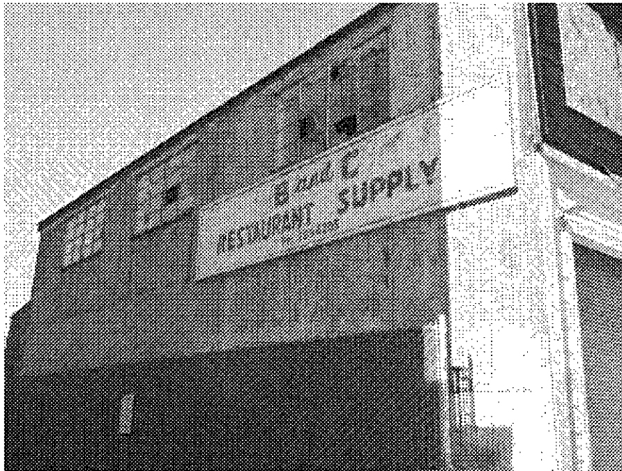
2nd Street and Franklin: broken windows, separated siding, peeling paint, and serious signage deterioration due to long-term neglect
