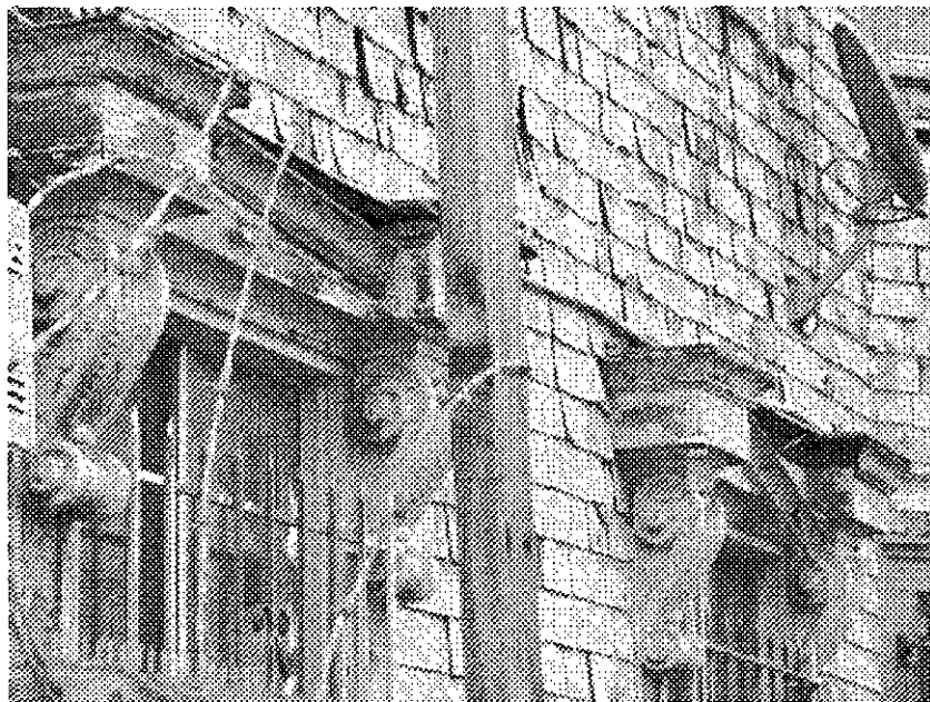
24th Street and Telegraph: deteriorated siding, substantial dry rot, peeling paint
