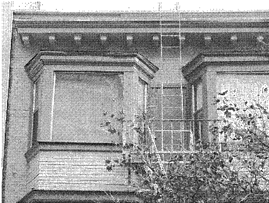
15th Street and Jefferson (close up of above): peeling paint, dry rot, deteriorated siding.
