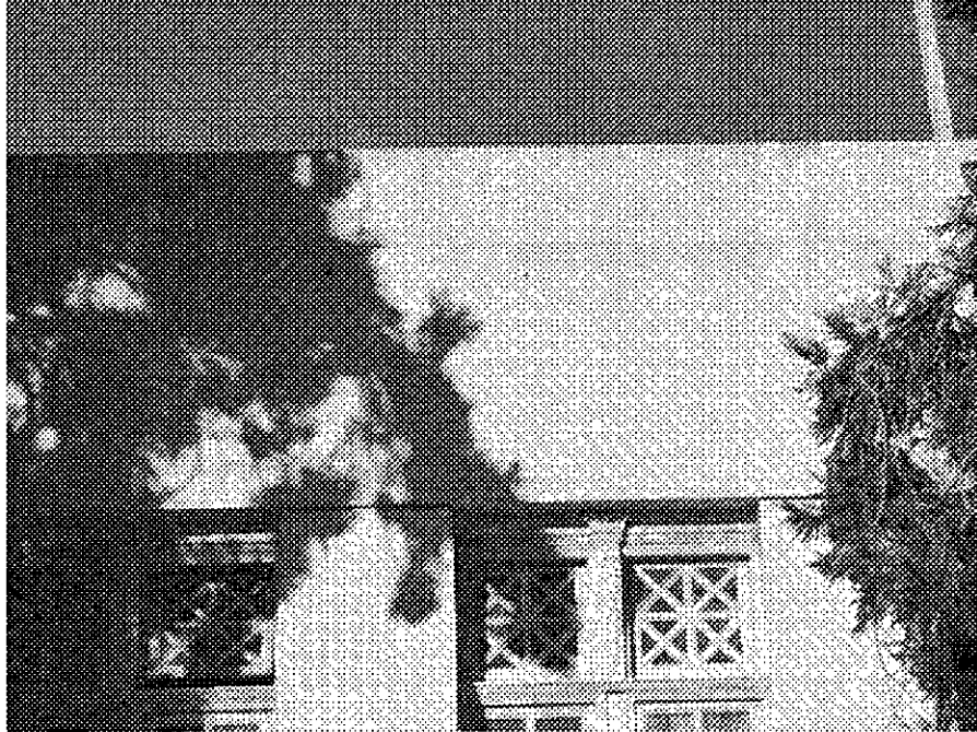
13th Street and Lakeside: cracked walls and peeling paint apparently due to long-term neglect.
