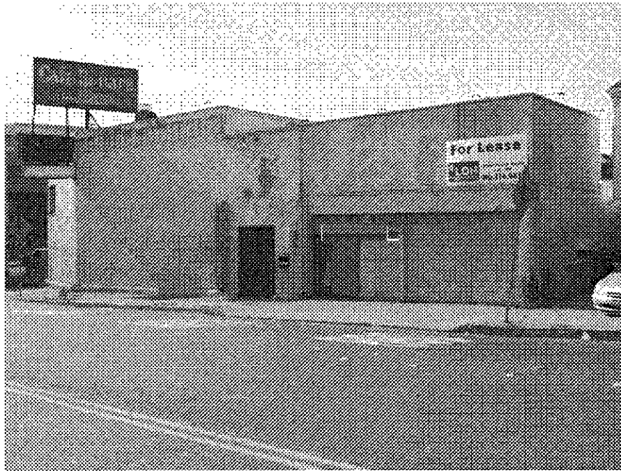
6th Street and Jackson: vacant commercial building with vandalism, partially reinforced masonry building vulnerable to serious damage from seismic events, potentially hazardous in event of earthquake.
