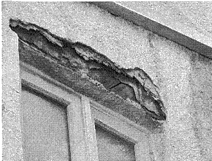
15th Street and Jackson (same building as previous photo): deteriorated siding likely allowing moisture intrusion, mold contamination and structural wood rot.
