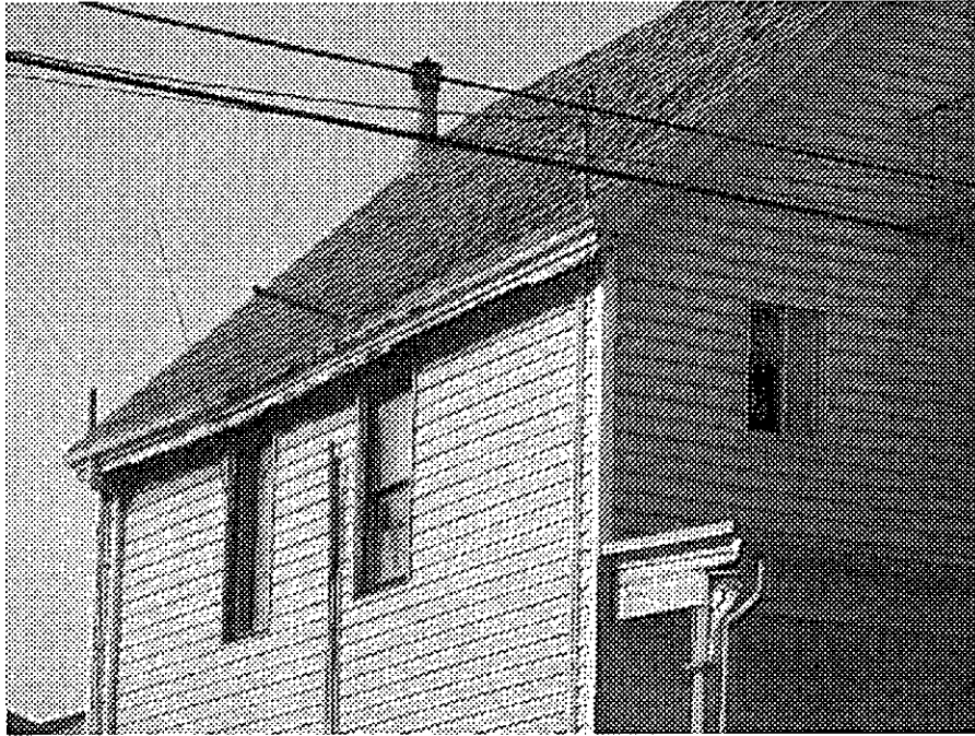
9th Street and Martin Luther King: severe roof dilapidation likely allowing moisture intrusion, mold contamination and structural wood rot.
