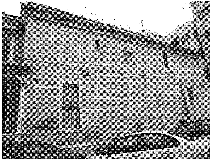
15th Street and Jefferson: deteriorated siding, peeling paint boarded windows, and cracked wall apparently due to long-term neglect
