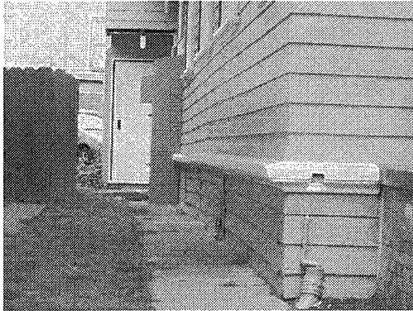
23rd Street and Harrison: structural alignment problems observed in building siding.
