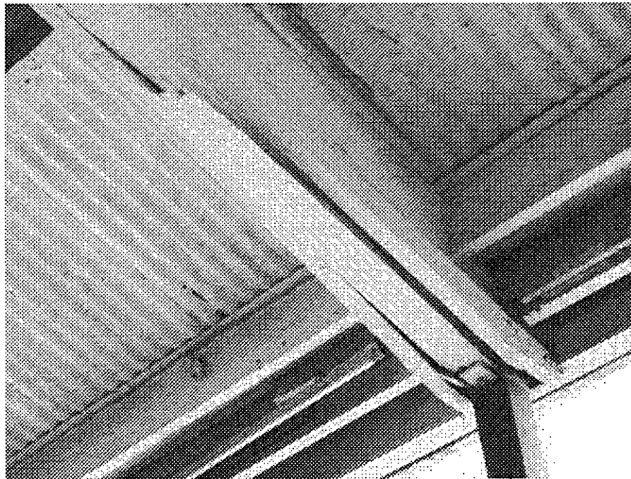
2nd Street and Franklin: deteriorated structural support, peeling paint, dry rot.
