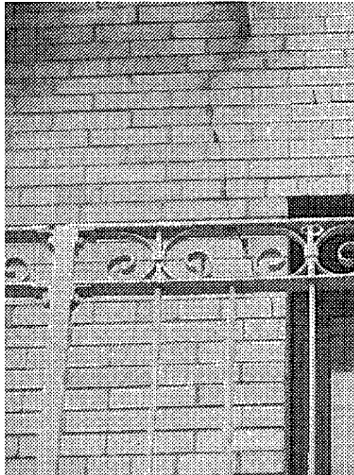
14th Street and Alice: cracked masonry wall potentially hazardous in event of earthquake, building vulnerable to serious damage in event of earthquake.
