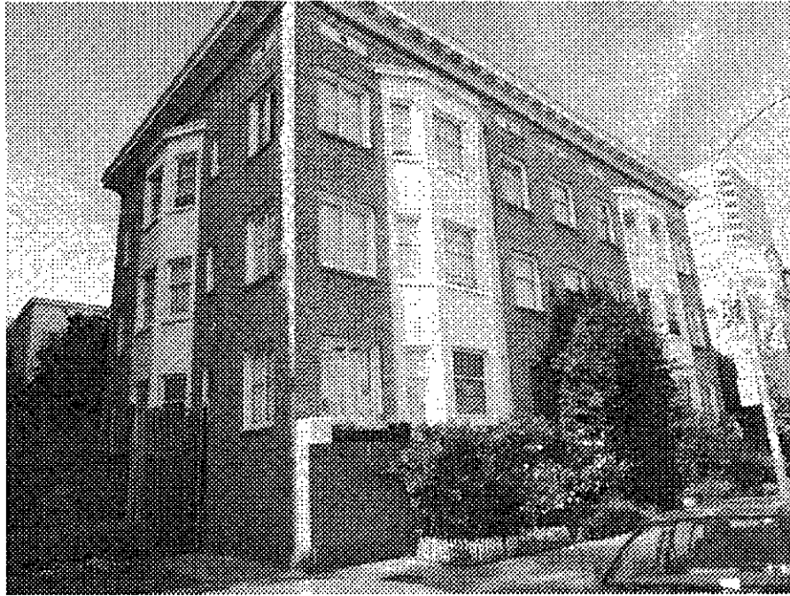
17th Street and Alice: masonry building vulnerable to serious damage from seismic events, building potentially hazardous in event of earthquake.
