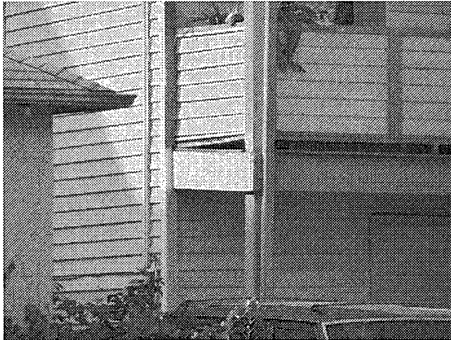
9th Street and Martin Luther King (same building as previous photo): structural alignment problems observed at porch.
