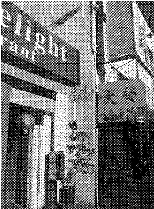
7th Street and Webster: cracked wall, peeling paint, evidence of vandalism on wall and awning.
