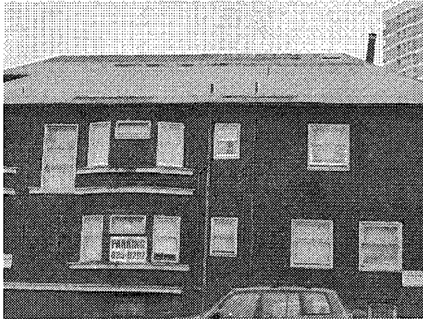
24th Street and Waverly: severe roof deterioration likely allowing moisture intrusion, mold contamination and structural wood rot.
