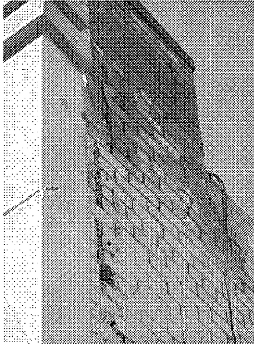
15th Street and Franklin (same building as previous photo): cracked masonry wall and separated facade potentially hazardous in event of earthquake, building vulnerable to serious damage from seismic events.
