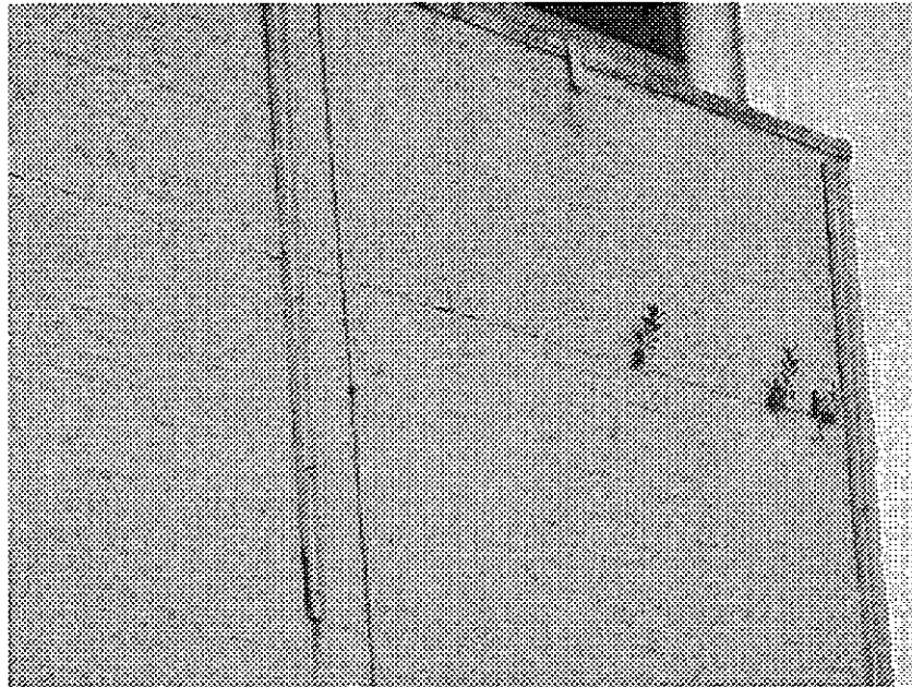
Grand and Valdez: unreinforced masonry building vulnerable to serious damage from seismic events, cracked masonry wall potentially hazardous in event of earthquake.
