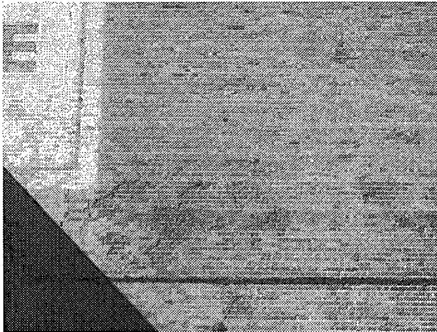
2nd Street and Clay: cracked and deteriorated masonry wall potentially hazardous in event of earthquake, building vulnerable to serious damage from seismic events.
