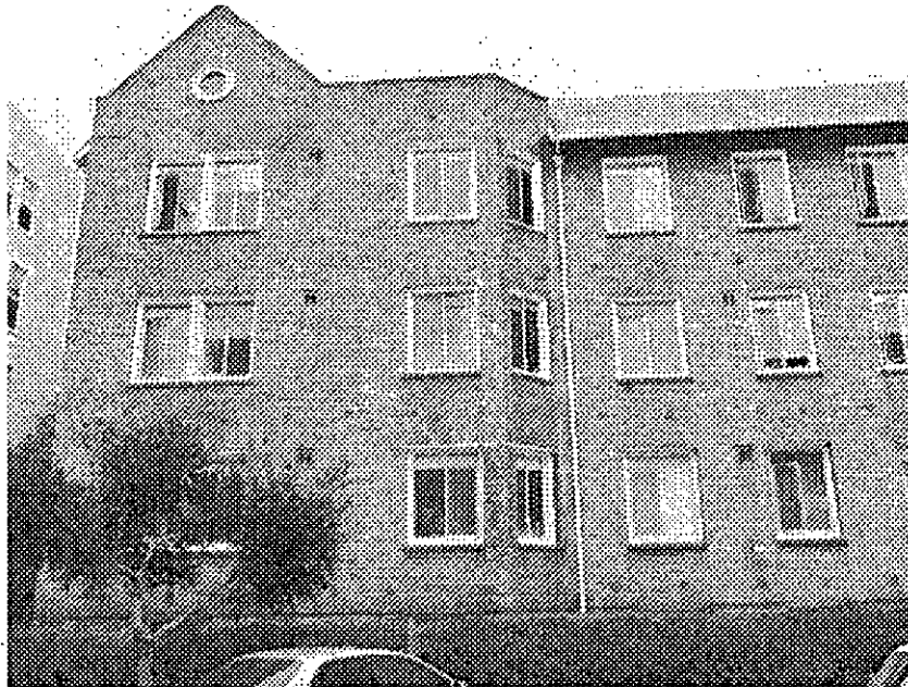
Bay Place and Access Road: partially reinforced masonry building vulnerable to serious damage from seismic events, cracked masonry wall potentially hazardous in event of earthquake.
