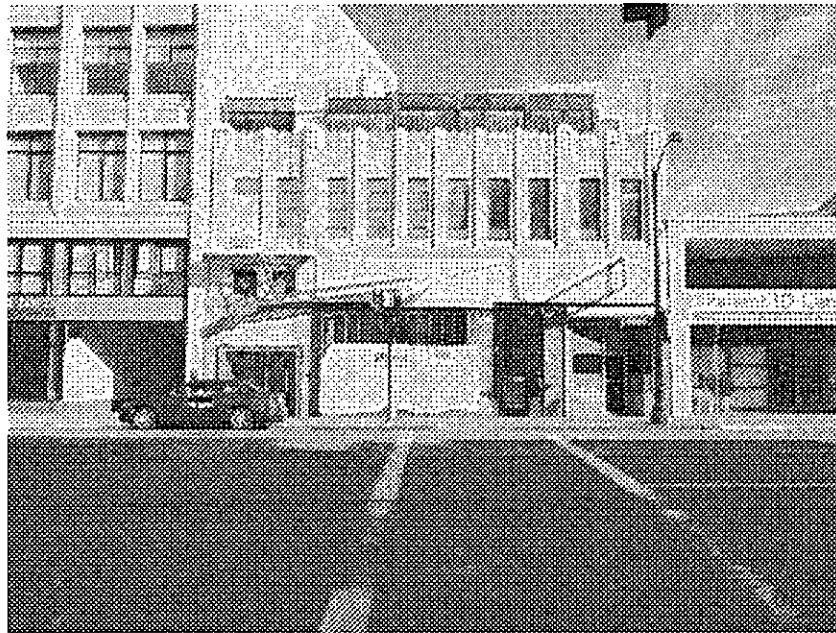
18th Street and Telegraph: unoccupied commercial building, missing and boarded windows, worn facade.
