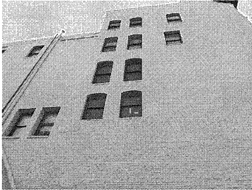
16th Street and Martin Luther King: partially reinforced masonry building vulnerable to serious damage from seismic events, building potentially hazardous in event of earthquake.
