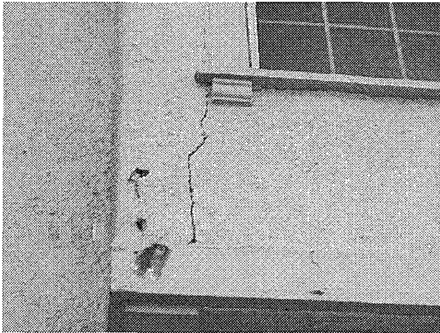
15th Street and Jackson (same building as previous photo): cracked wall.
