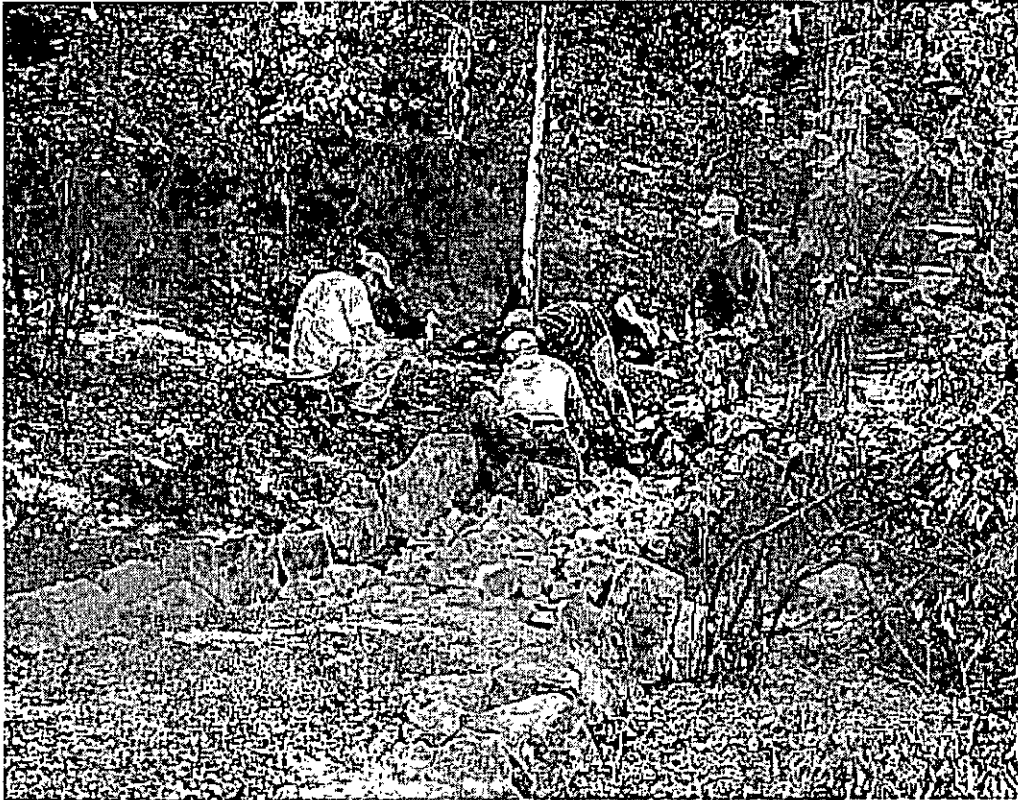
After fitting in the boulders and rock by hand like a 3-dimensional jigsaw puzzle, gravel was added on top to help with drainage and to make it safer to cross.
