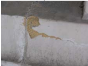
MINOR SURFACE SPALL - COAT EXPOSED BRICK
