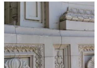
MINOR SPALLS PATCH AND COAT
