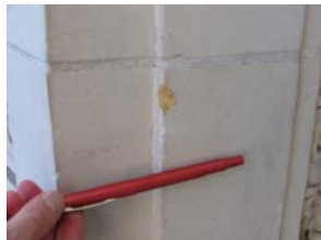
VERY MINOR SPALL - COAT EXPOSED BISQUE
