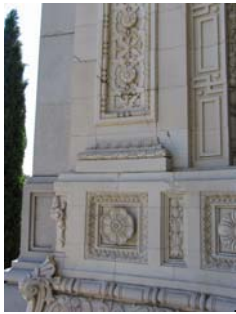
LARGE CRACK: PATCH - POSSIBLE UNIT REPLACEMENT
