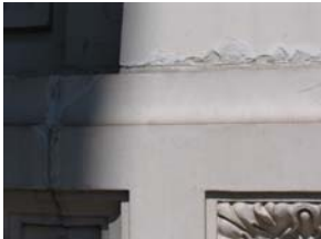
PREVIOUS BAD PATCH - REPLACE
