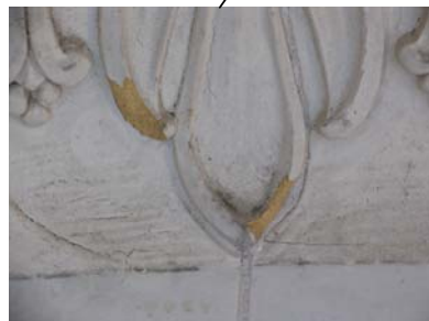
MINOR SPALLS - PATCH AND COAT
