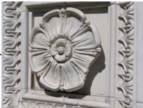
SPALLED ROSETTE - COAT BROKEN EDGE
