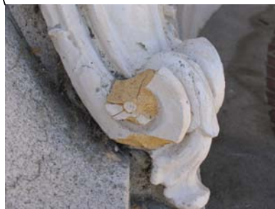
SPALLED CORNER PIECE - COAT BROKEN EDGES
