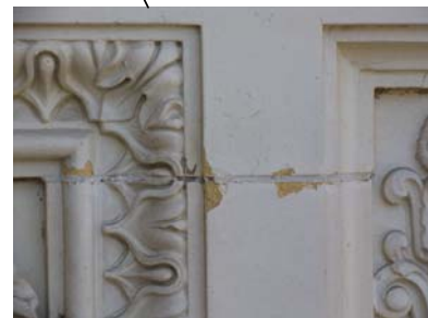
MINOR SPALLS - PATCH AND COAT
