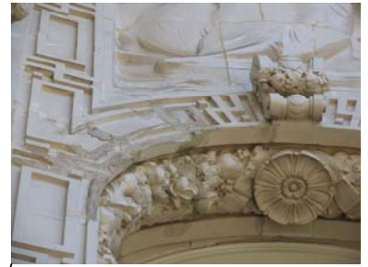
BAD PATCH - REPLACE
