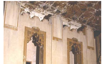
Fox Theatre interior damage
