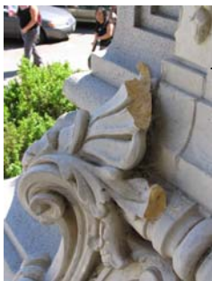
SPALLED CORNER UNIT COAT BROKEN EDGE
