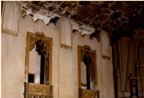
Fox theatre interior damage
